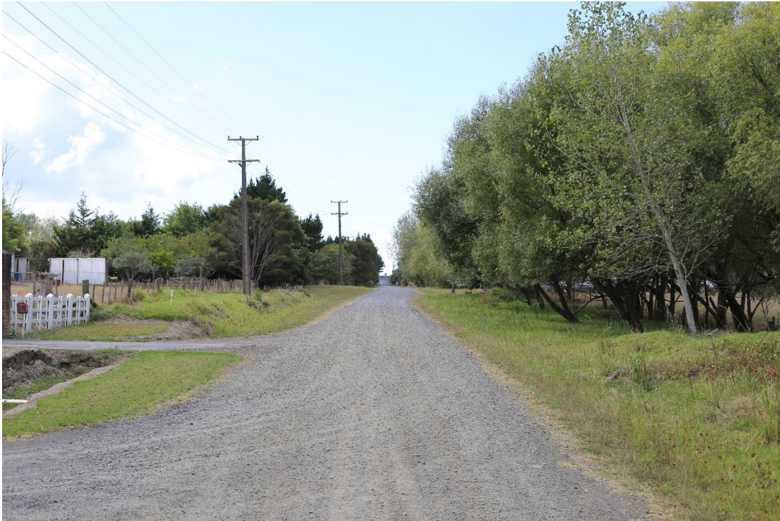
Plate 10. View of Spedding Road condition (looking east)
