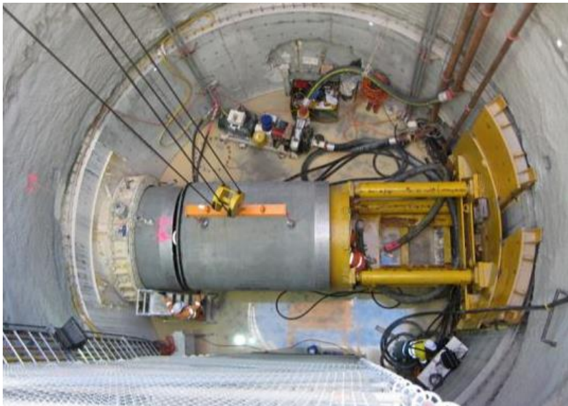
Figure 3-14. Earth pressure balance TBM including hydraulic jacking frame.
