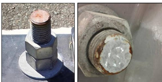
Figure 2: Examples of threaded rod corroding where it has been cut to length.
