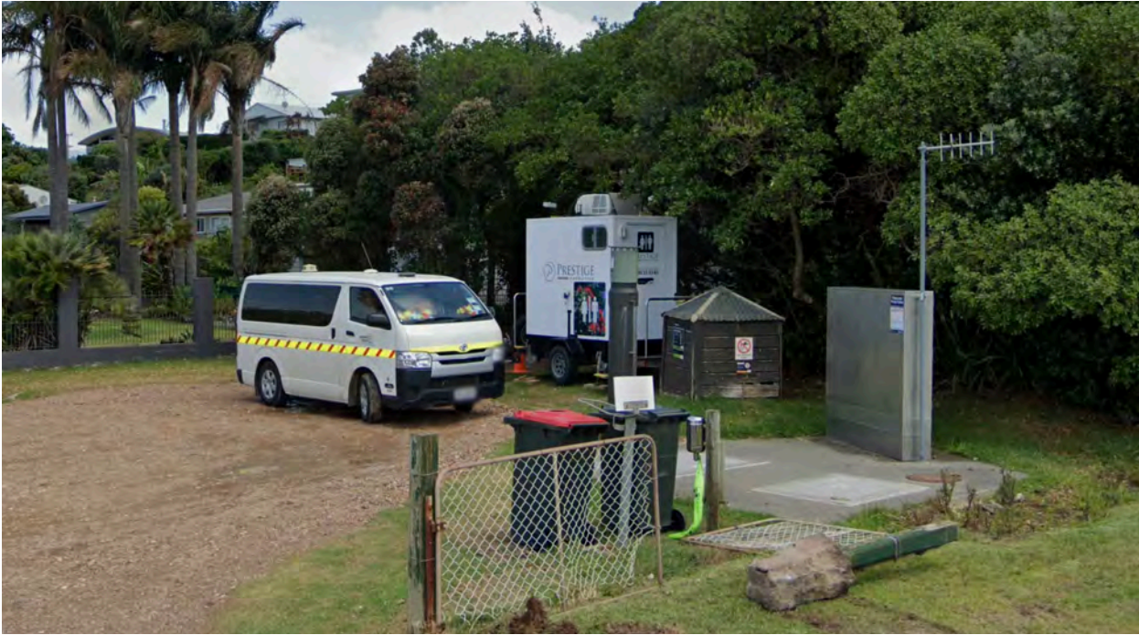
Figure 10 – Oneroa Pump Station (Source: Google Streetview)
